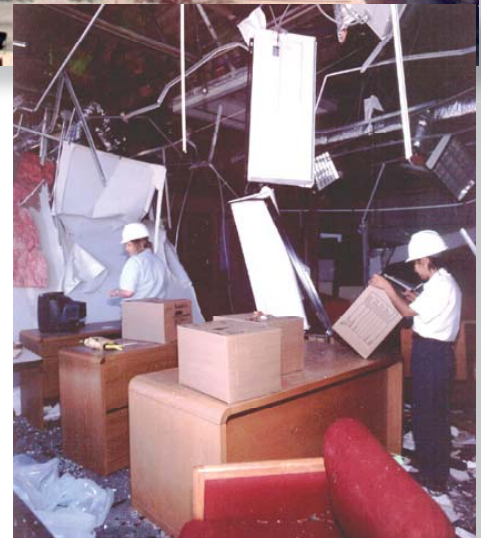
Texas Tornado Damage
